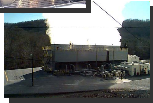
New cooling tower
