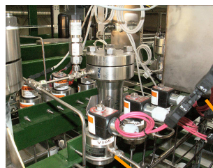
Impurities dosing system
