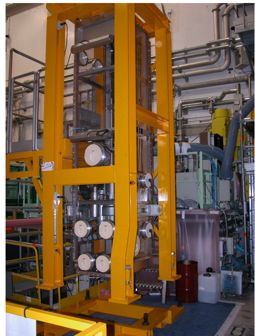
Photo 16: Glove box for in-service inspection
