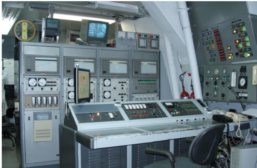
control room view- 2007
