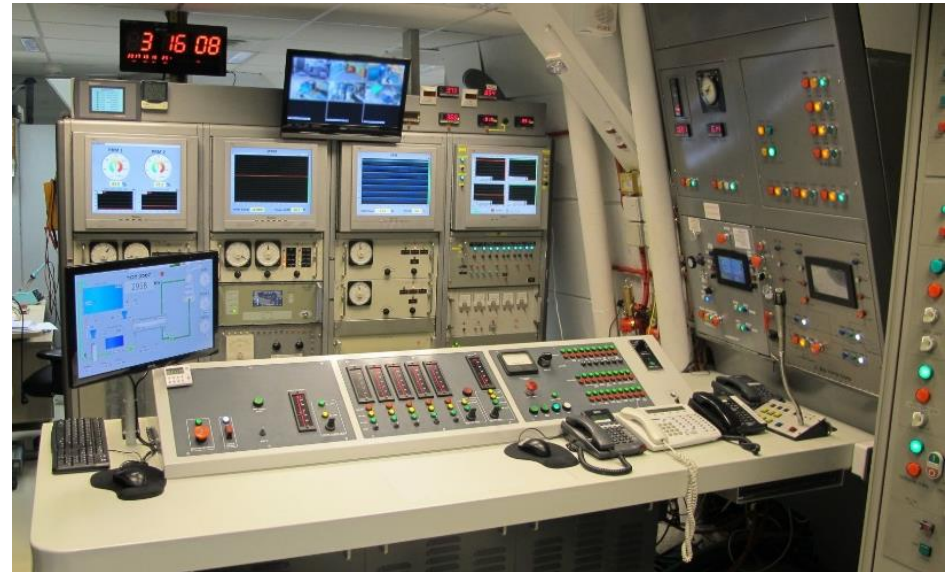
control room view- 2017
