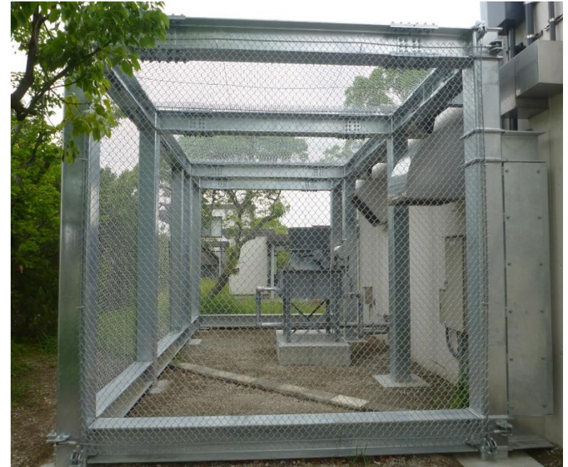
Protection Cage for Cooling Tower of Emergency Generator (EG1)
