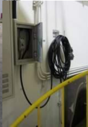
Emergency power supply line
