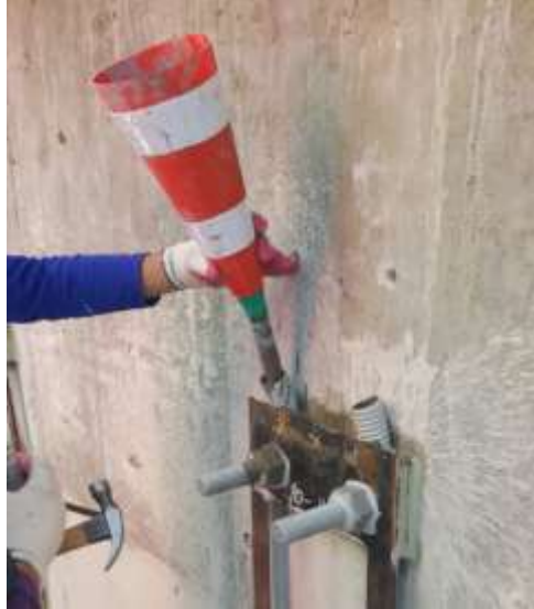
FIG. 9. Inject non-shrink grout into hole to fix the through bolt in the hole.
