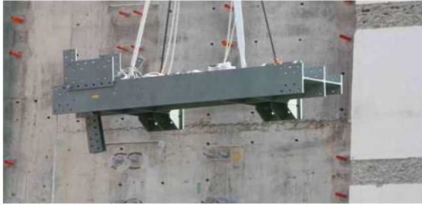
FIG. 11. Crane is lifting the built-up section to install with through bolt at the wall
