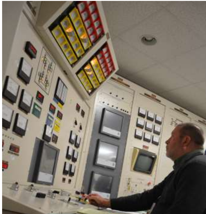
FIGURE 4. TREAT control room simulated operations
