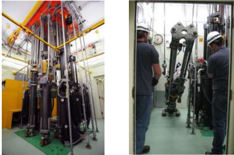
FIGURE 2. TREAT Subpile room showing the control rod actuators and replacement activity
