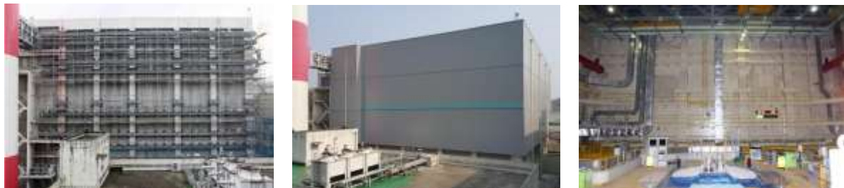
(a) Exterior installation
