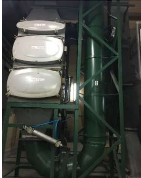
FIG. 6. Emergency ventilation system
