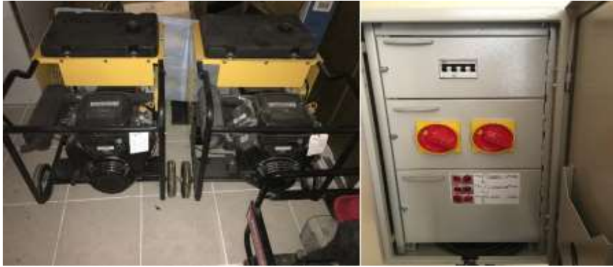
FIG. 4. Emergency generators and the connection box
