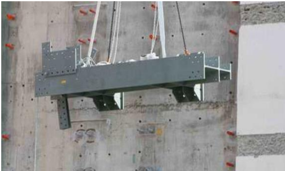
Crane lifting the built-up section to install with through bolt at the wall
