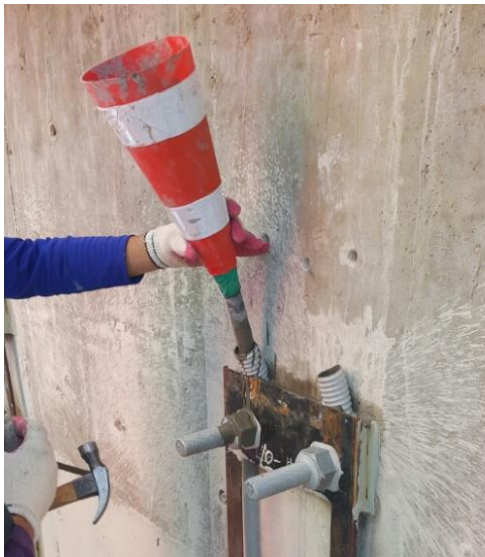
Inject non-shrink grout into hole to fix the through bolt in the hole
