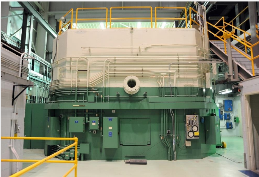
South View of the Reactor
