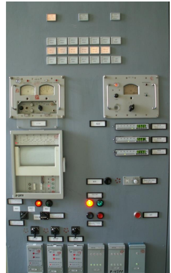
3 rd control channel and backup control board
