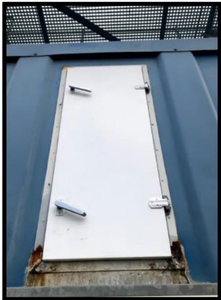
Original: corroded access door
