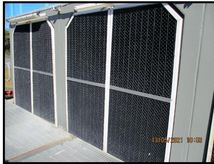
New Air Inlet Louvre Panel
