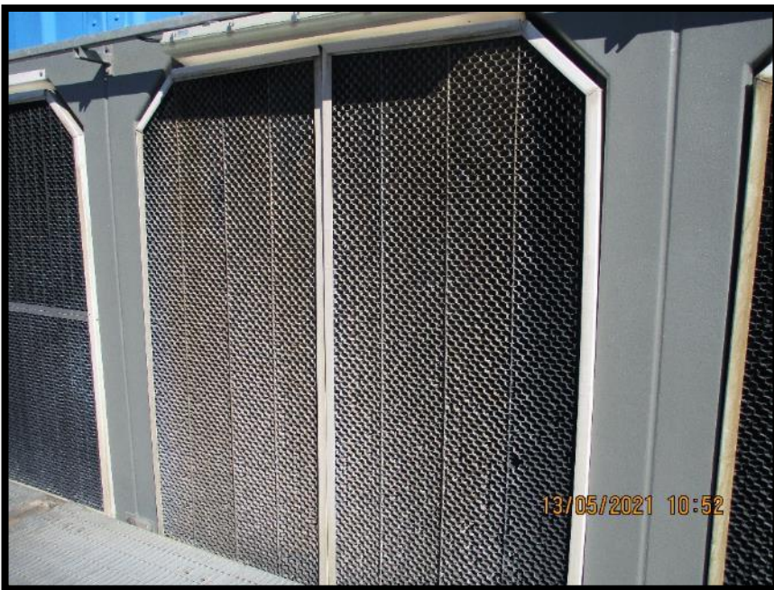
Old Air Inlet Louvre Panel
