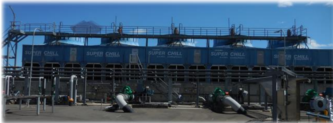
SCS Five module Cooling Tower
