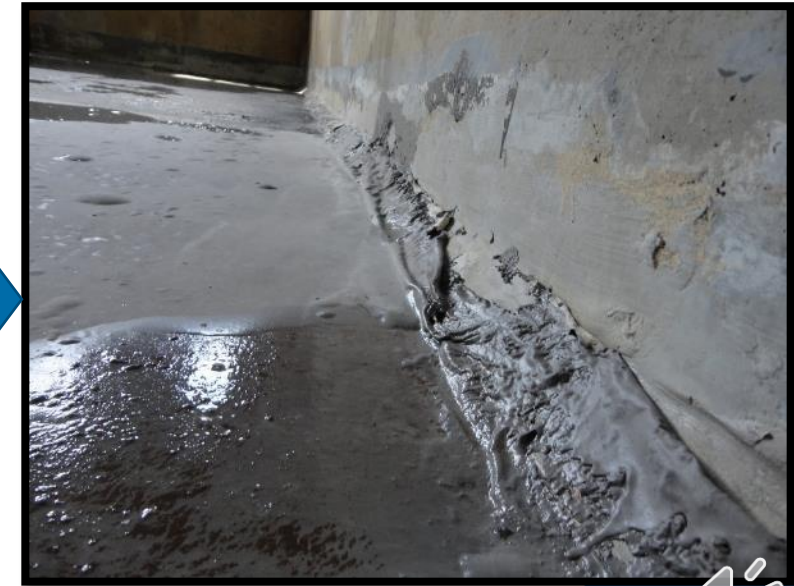
Failed Coating Remnants
