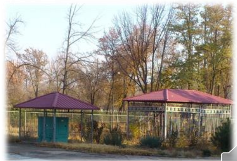
Transformers and 40 kW Diesel generator
