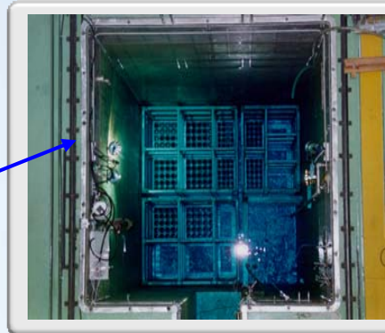
Spent Fuel Storage Pool
