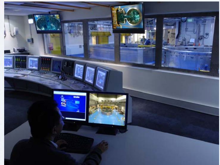
View of the Control Room and the Reactor Hall from Shift Manager's desk
