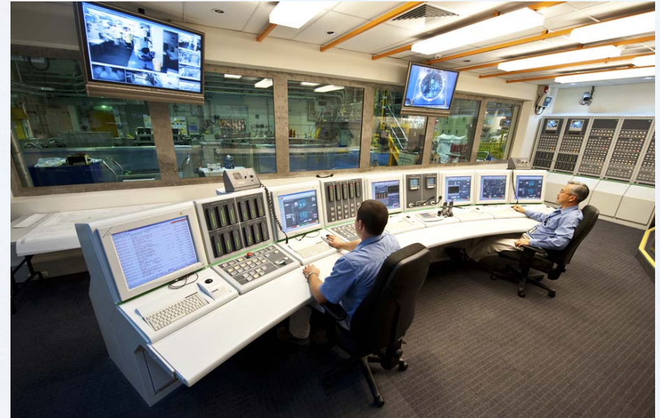
OPAL Control Room – looking out to the Reactor Hall
