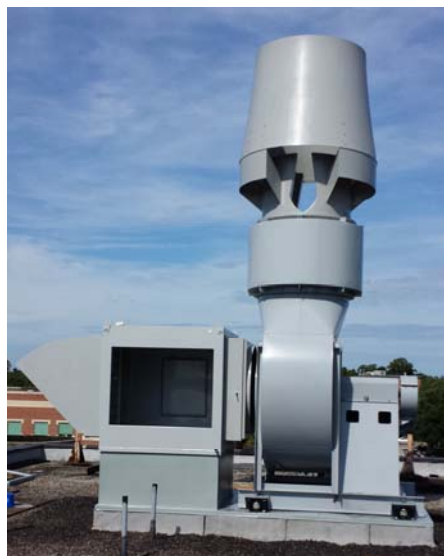
Fig 2: The high-plume exhaust fan and monitoring equipment as installed.
