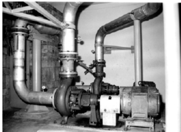
Fig. 5 Modified pipe support
