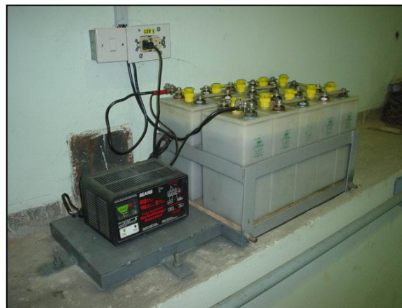
Fig 6b: ECCS Battery & Charger unit
