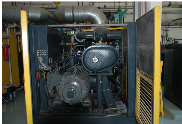
Fig. 1 Helium Compressor used in the CNS Cryogenic System
